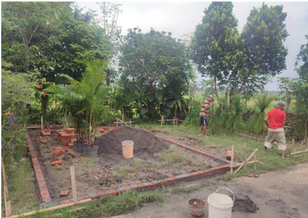
Figure 2. Location of Land to Move Old Mosque to be Demolished in Griya Salam
